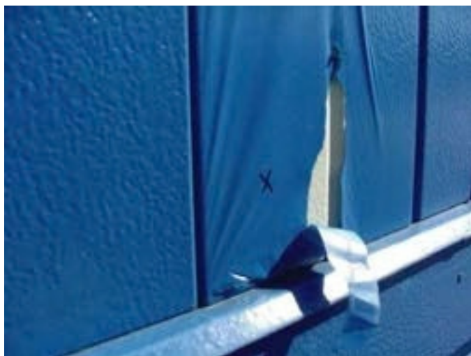
Figure 48. The topcoat delaminated from the primer.
