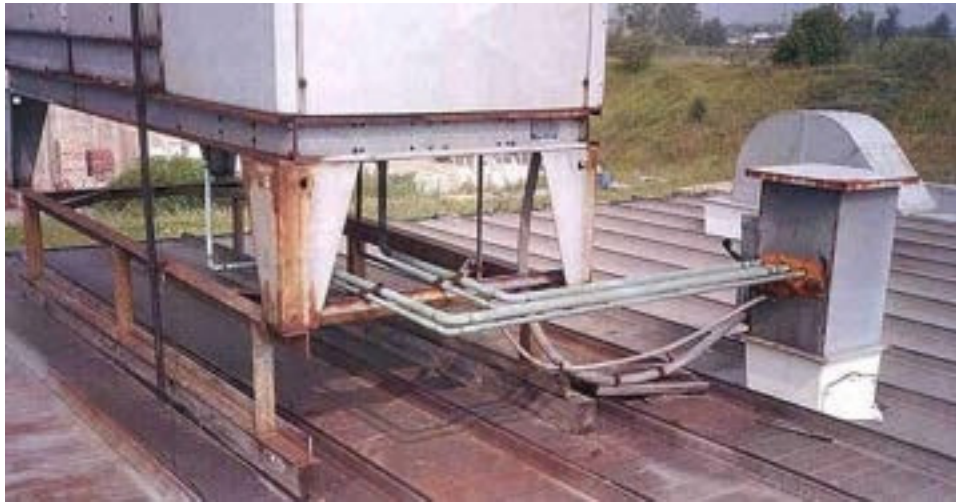
Figure 36. GALVALUME® roof panel corrosion due to condensation water runoff from the copper pipes.
