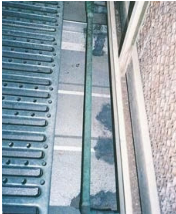
Figure 37. GALVALUME® panel corrosion due to condensation water runoff from the copper pipes.
