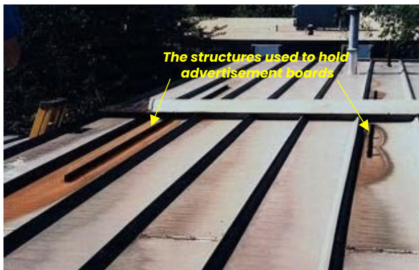
Figure 23. Photograph of a GALVALUME ® roof after 21 years service. The localized corrosion was caused by water ponding at the low spots where the advertisement boards were set on top of the roof.
